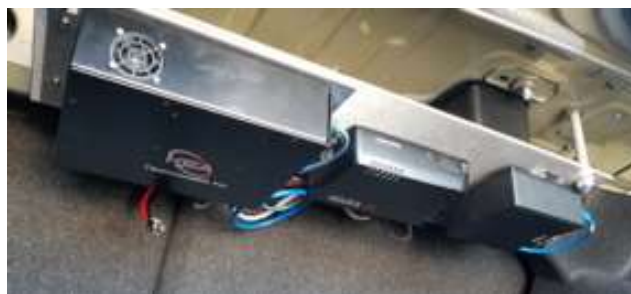
Figure 15. Equipment located in the trunk, from left to right, DAS, WIFI LTE, network switch, and DVR
