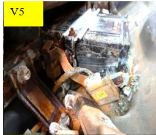
12V battery & surrounding
