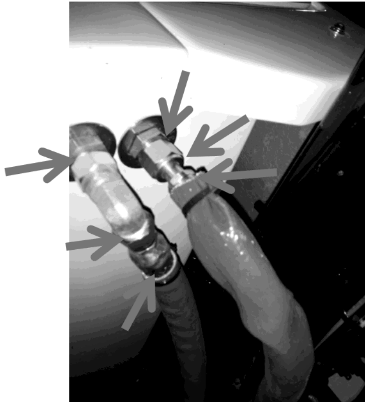
Figure 9 When looking for hose leaks, check the hose-to-fitting junctions as well as fittings as indicated by the arrows. Move additional protection (fire sleeve) if necessary for access.
