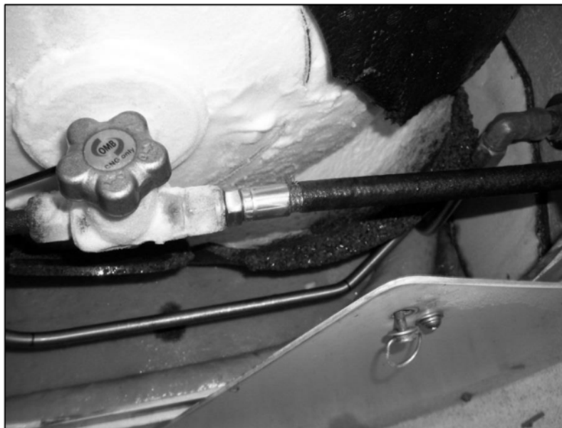
Figure 4 Frost forming near a CNG gas leak. The leak is located at the junction of the braid and fitting ferrule.
