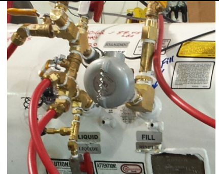
C. Nitrogen temperature in the tank is monitored.
