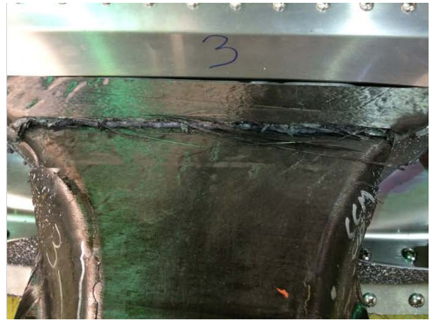
(b) Damage at the Hat Root
