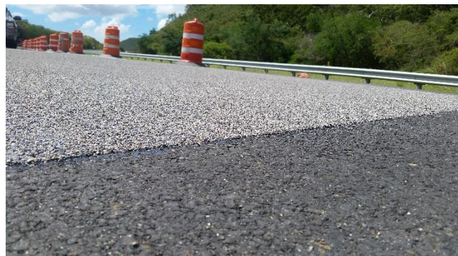
Implementation of the High Friction Surface treatment in the PR-54 with PR-7711.
